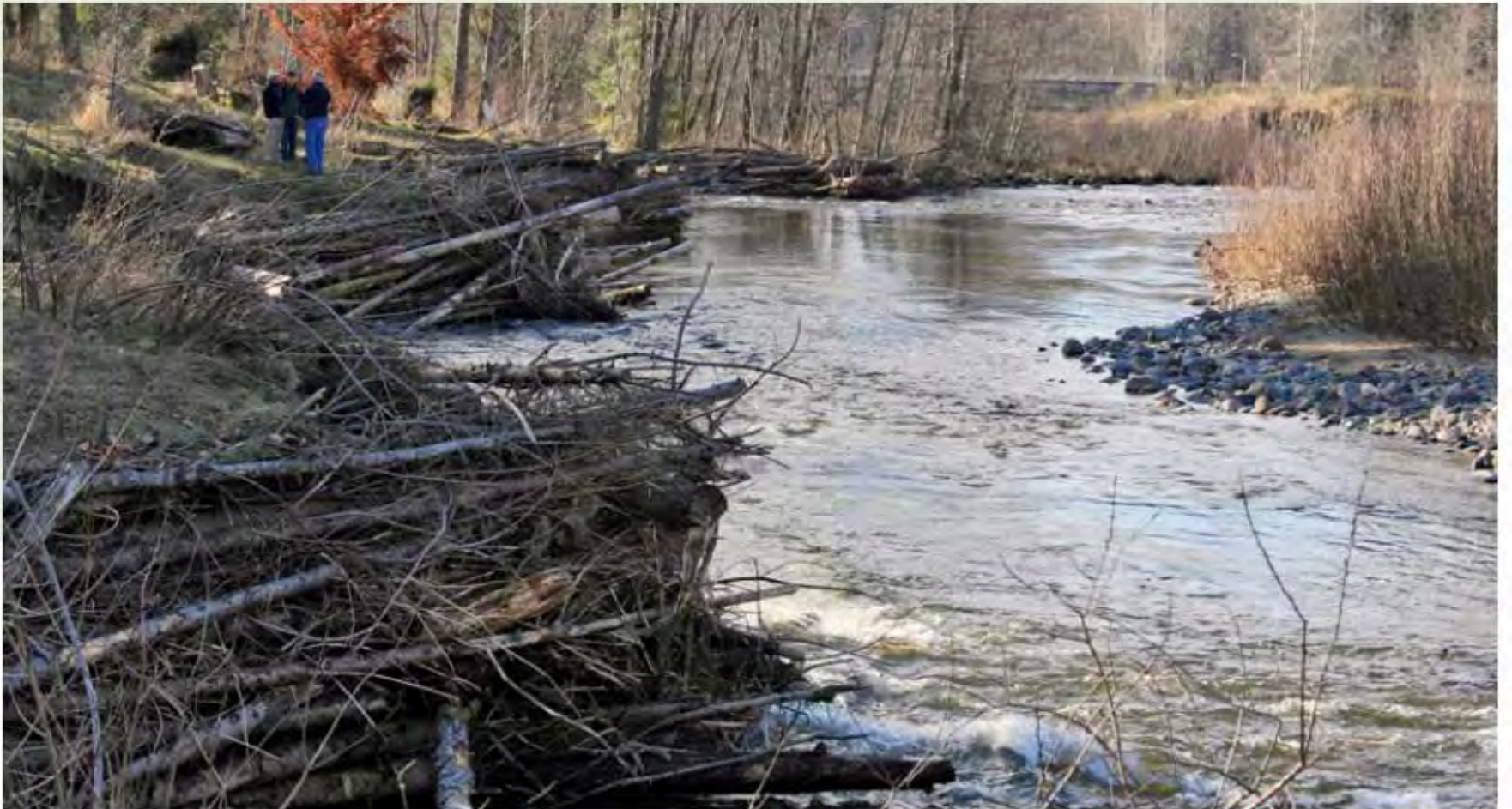
Four of the engineered logjams designed by Herrera Environmental Consultants on the Mashel River outside of Eatonville, WA.
