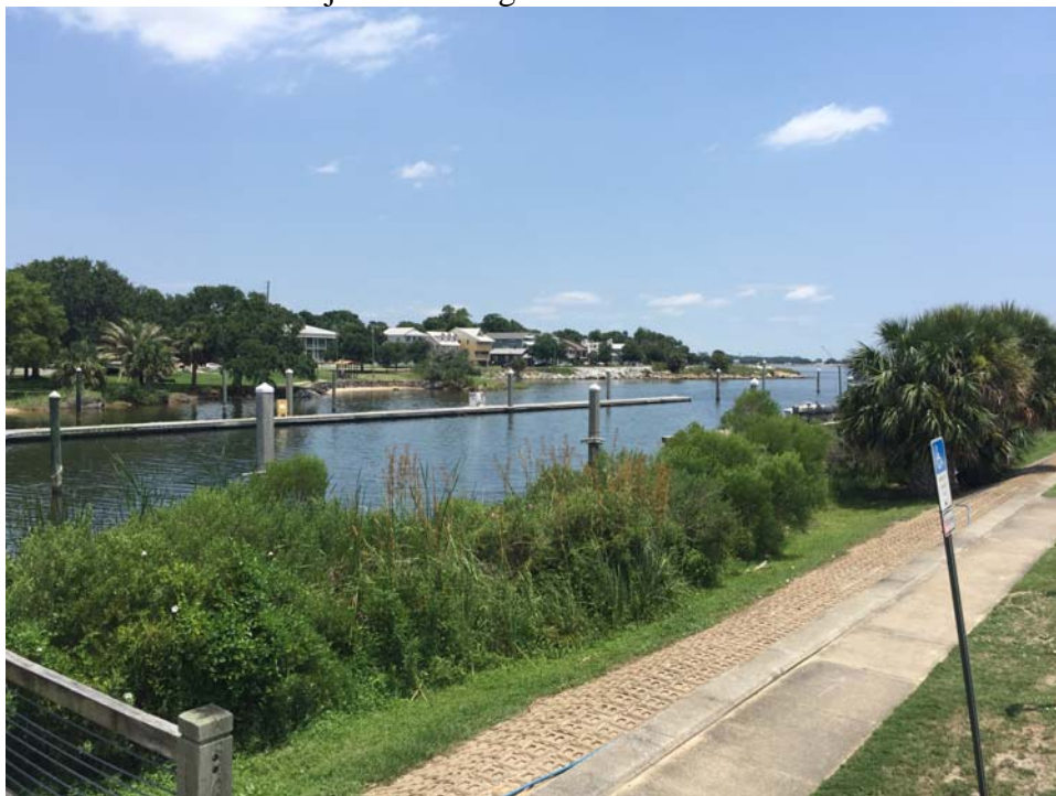
View of Existing Damaged Floating Dock
