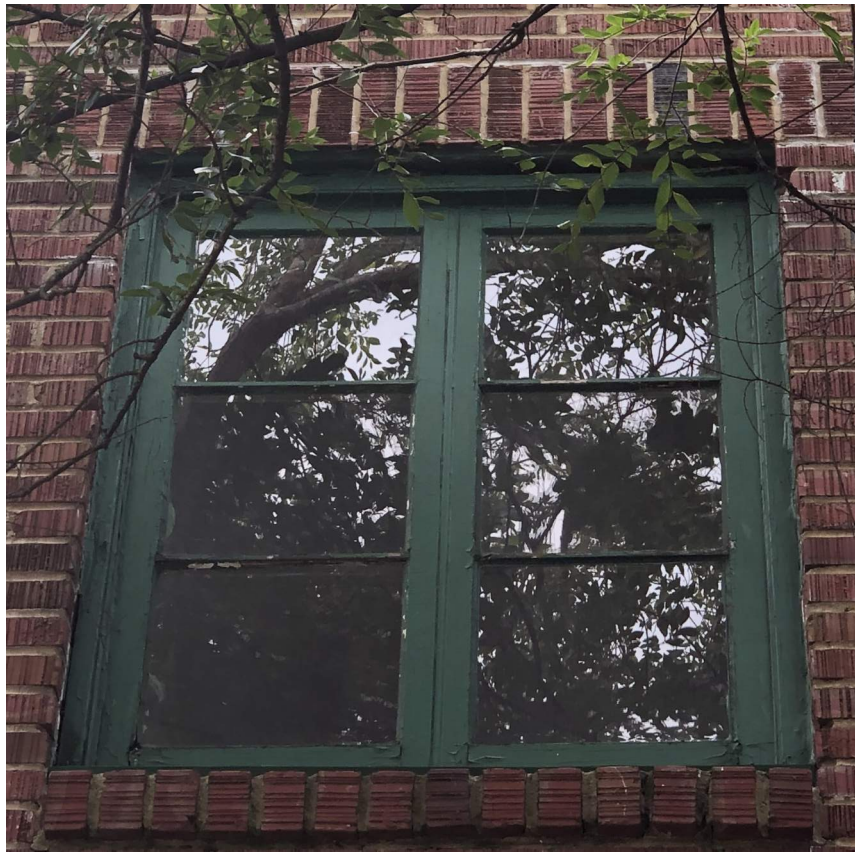
EXISTING UPPER WINDOW TO BE REPLACED (EXTERIOR VIEW)
