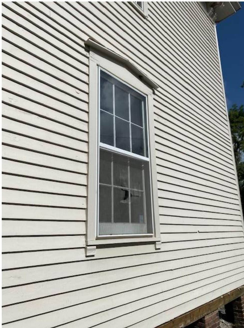
226 Government Existing Window and Trim Condition
