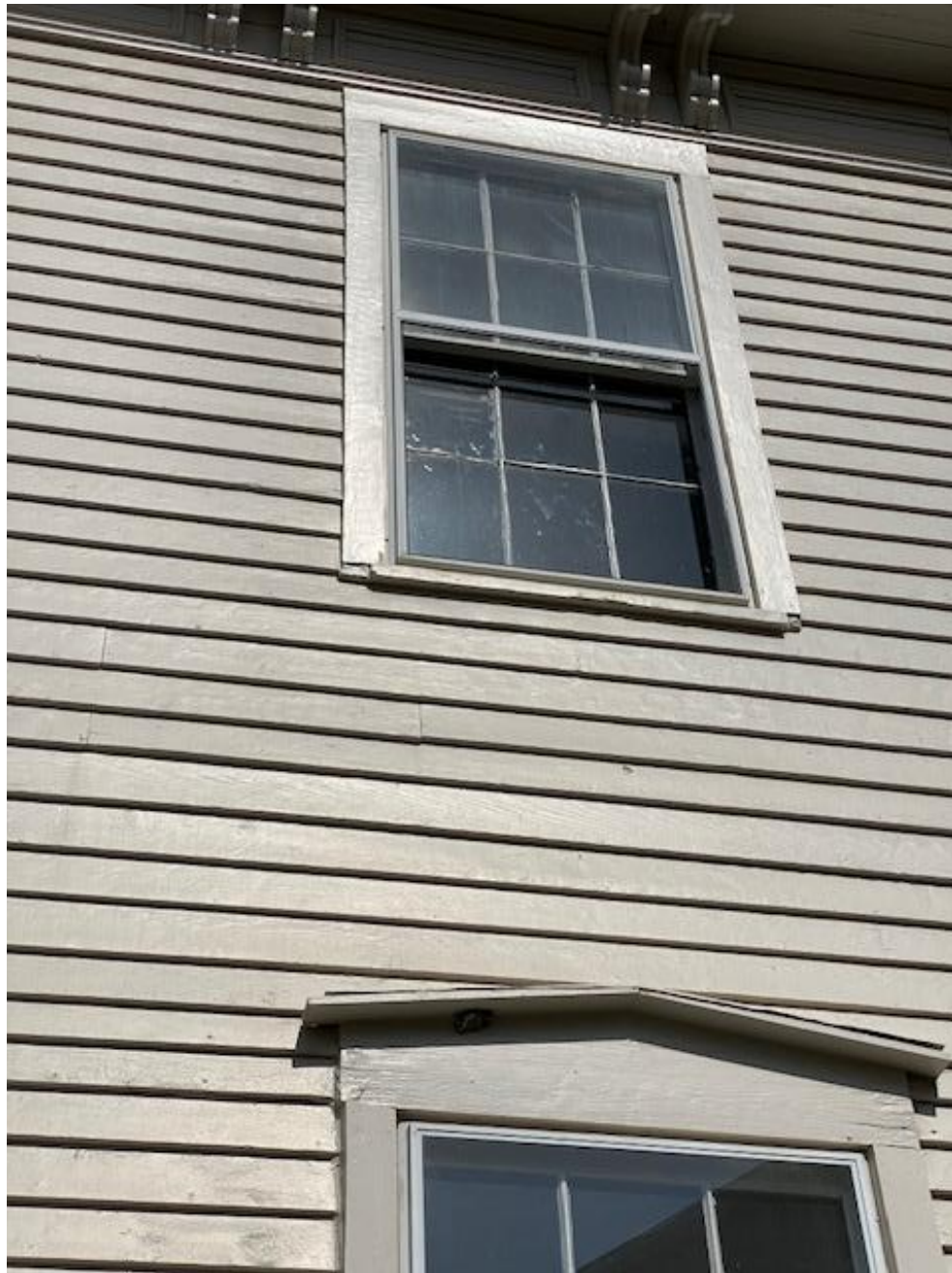
226 Government Existing Window and Trim Condition
