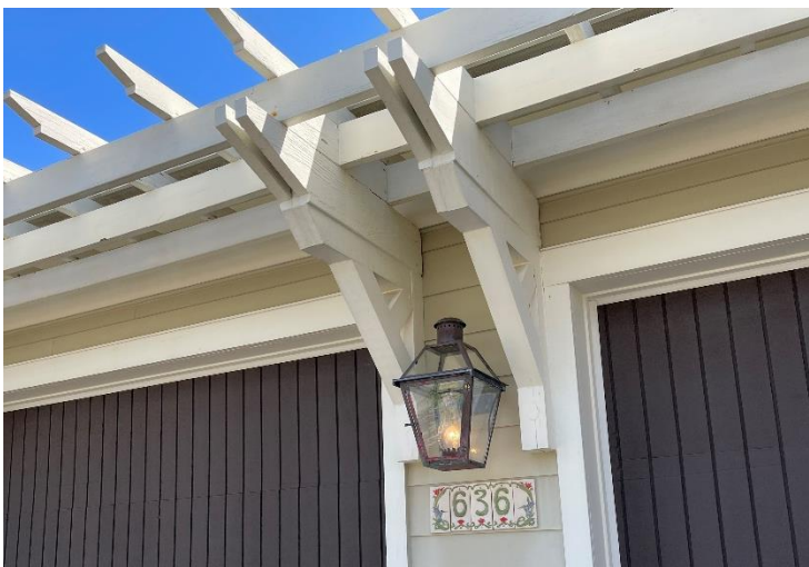
EXISTING BRACKET @GARAGE
