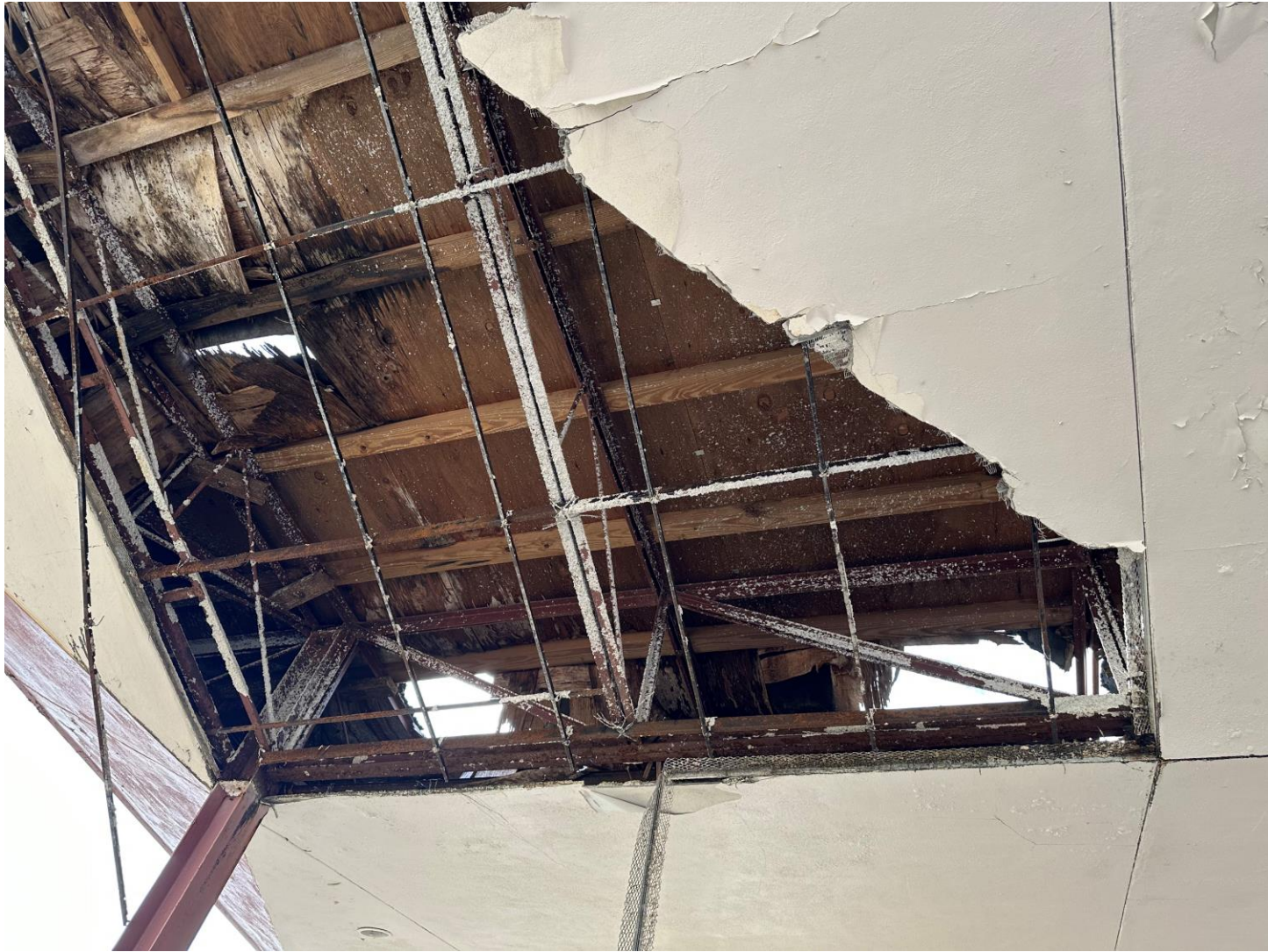
Immanuel Lutheran Church Overflor parking Failing structure view
